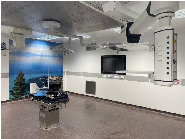
Last generation integrated Operating rooms
